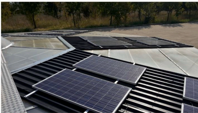
(b) Close-up view of PV panels installed on the solar updraft tower's collector
