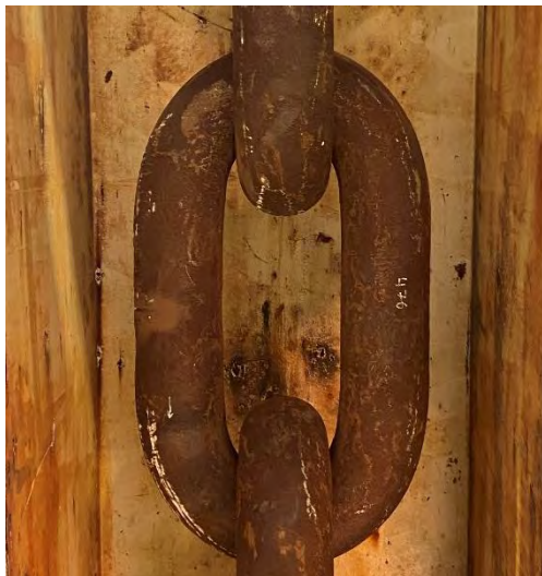
Figure 1: Mooring chain sample showing corrosion
