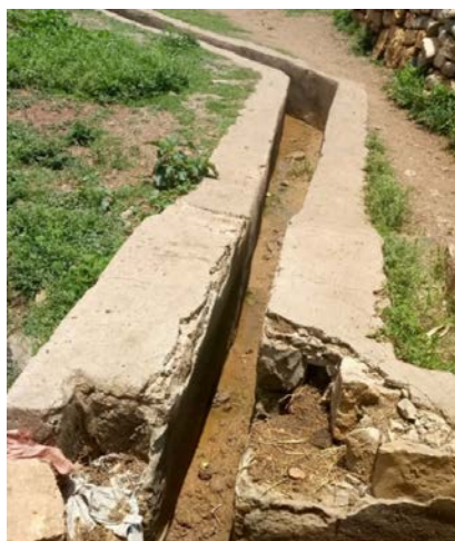
Figure A2. Poor canal maintenance at the Shilant-2 dam; the photo was taken by A.A.M. on 21 August 2019.
