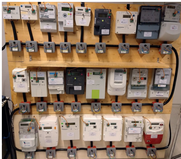
Figure 3.2. Picture of the 24 static energy meters placed in series in the setup.
