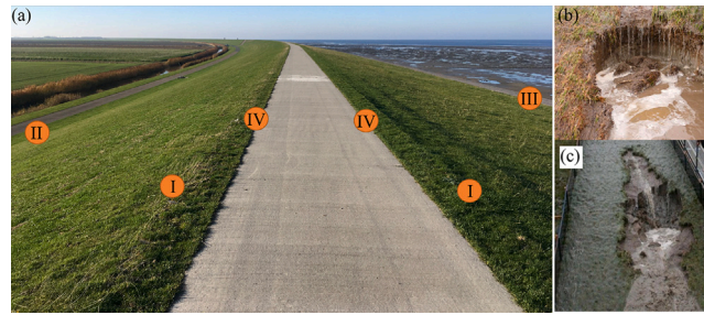
Fig. 1. (a) A photo indicating transitions in cover type (II, III, IV), height (IV) and slope (I, II, III) on a grass-covered flood defence with roads on the crest and at the landward toe located at the Wadden Sea in the Netherlands. (b) Photo of a damage resulting in a small cliff (Bakker et al., 2008). (c) Dike cover erosion on the landward slope during wave overtopping field tests in the Netherlands.
