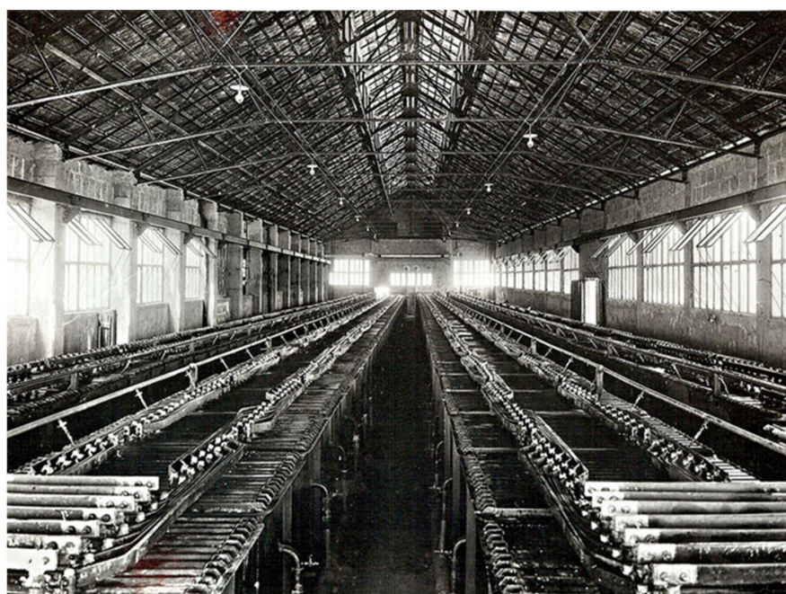
Figure 4. Electrolyzers in the Sabiñánigo ammonia factory in Spain, constructed in 1925. Courtesy Casale S.A.
