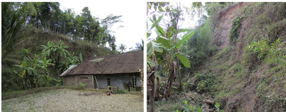
Fig. 2. Landslide on cut slopes in the built up area.
