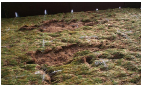
Figure 1. Example of a damage of the dike cover as the result of wave overtopping (Van der Meer et al., 2010).
