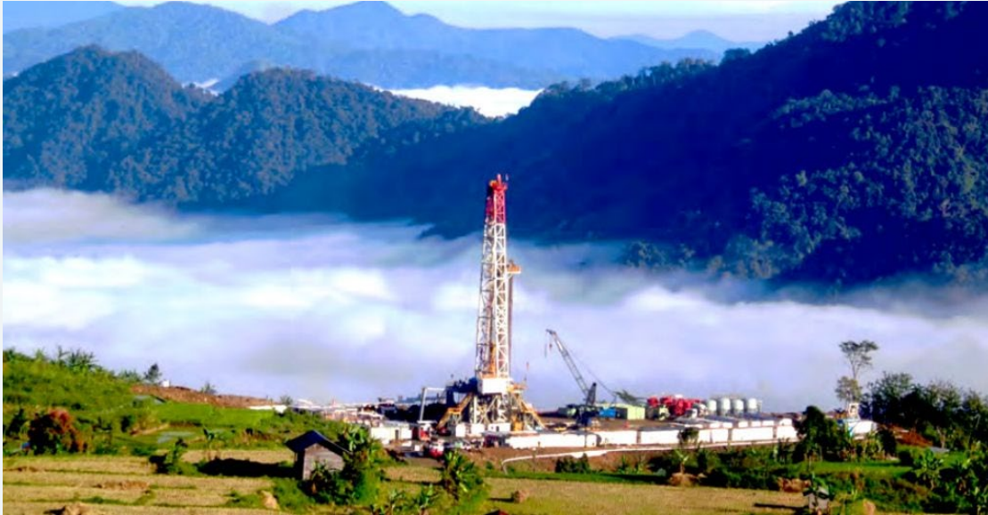
Muara Laboh geothermal power plant (Sumatra)
