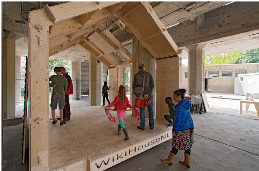
Figure 1: Example of a Wikihouse-structure: WikiHouseNL pavilion at the Meelfabriek-area in Leiden, Dag van de Architectuur 2014. Photograph by Jan Willem de Groot
