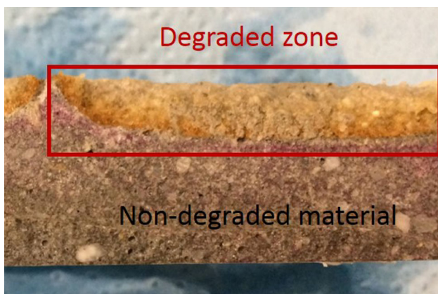
Fig. 1 Acidic deterioration in cementitious material. Cross-section of specimen subjected to degradation from only one side. Sharp transition between pristine and degraded material
