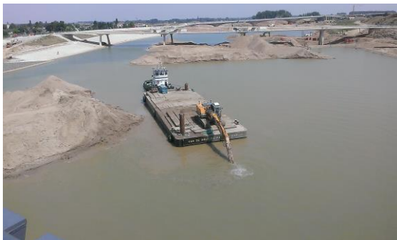
Figure 1. Excavation of flood channel along river Waal at Nijmegen under the Room-for-the-River programme.
