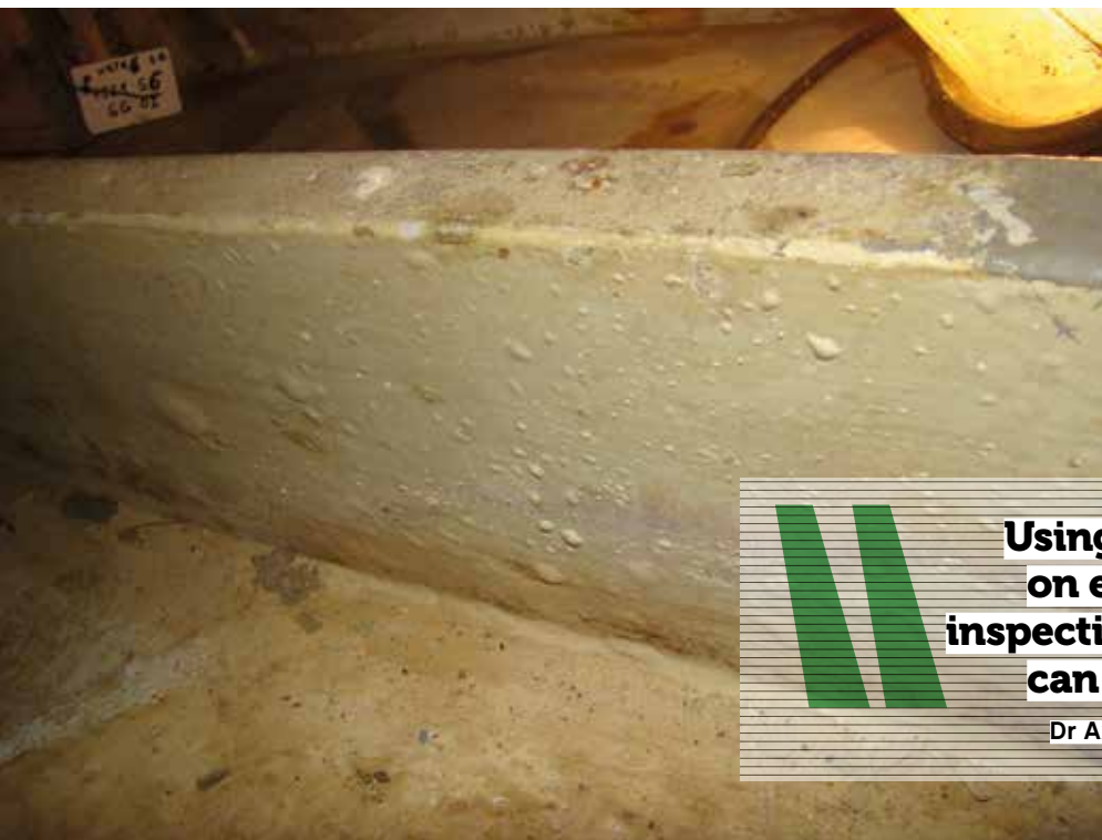
LEFT: Corrosion blisters underneath a protective organic coating inside a ship's ballast tank
