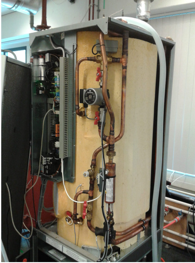
Figure 4.4 – Alpha-Innotec heat pump storage combination used for testing
