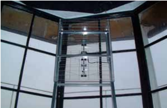
Figure 2-17: The antenna in the lantern room
