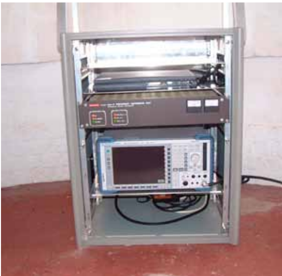
Figure 2-18: The equipment rack
