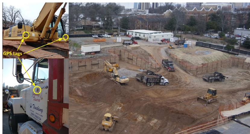
Fig. 4. GPS tags mounted on an excavator and a truck (left), data collection site (right).
