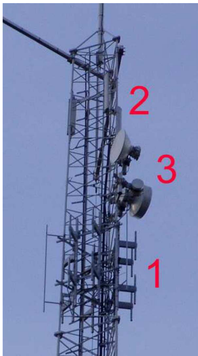
Fig. 11. Photograph of the top section of the mast where the DAB transmit antennas are mounted: 1 = band III antenna, 2 = L – band antenna and 3 = microwave dishes. Other installed equipment is property of the C2000 organization. (Photograph taken from http://www.radio.nl/fmvtv .)
