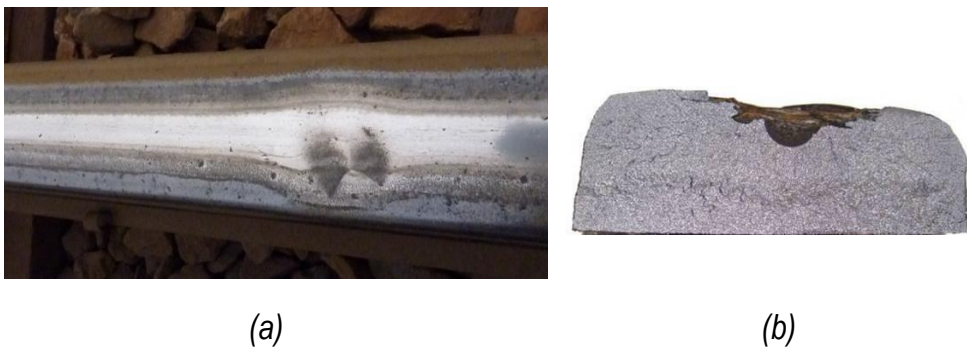
Figure 1.2 A typical severe Squat (a) and cross section of a Squat after four point bending (b).
