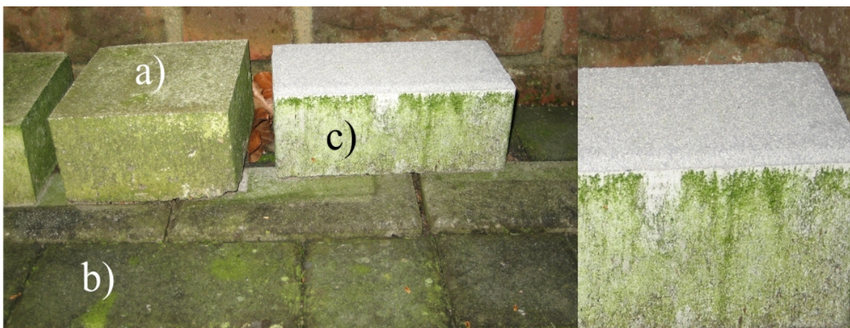
Figure 7: Staining of concrete paving blocks due to algae formation: untreated sample (a); paving of untreated paving blocks (b); paving block containing TiO 2 in the functional top layer (c)
