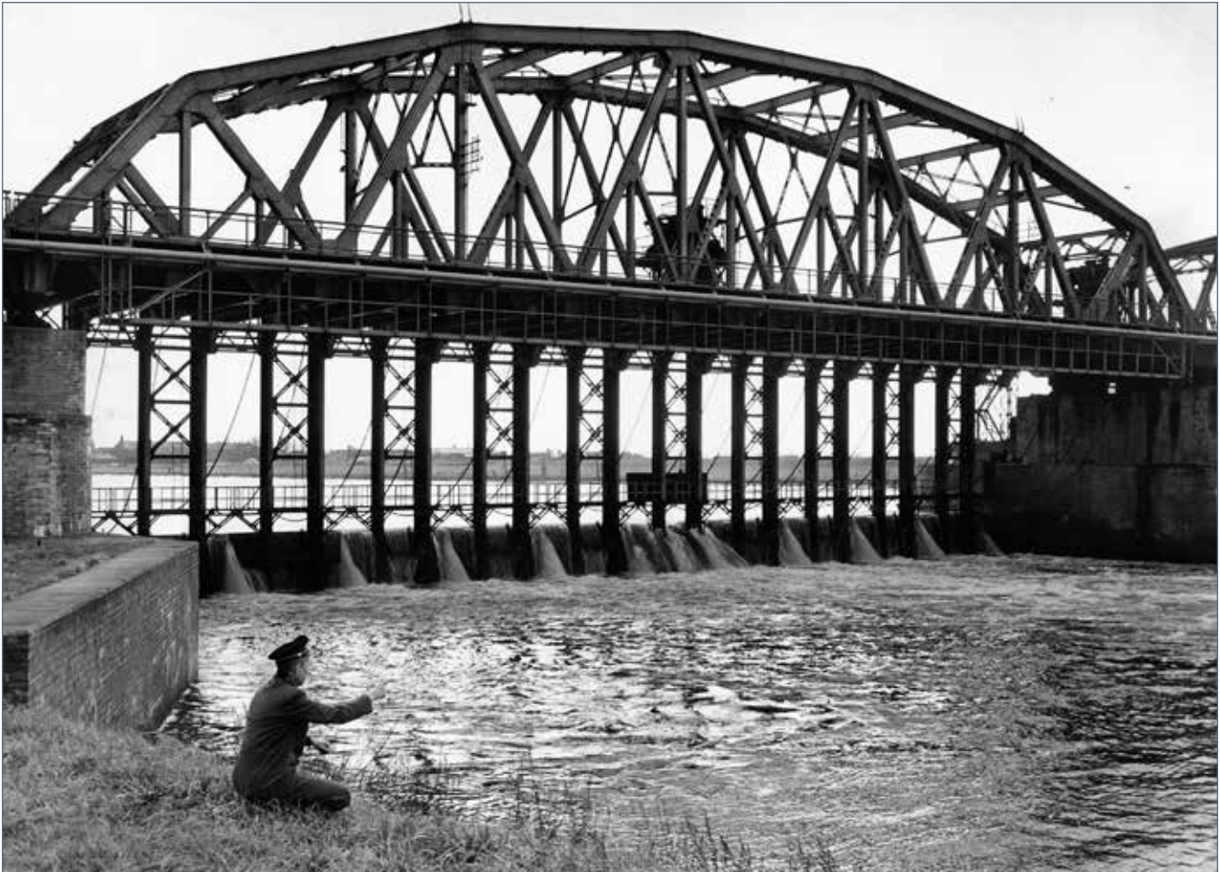
Weir at Grave, one of the weir construction projects in the Meuse canalization program, aimed at facilitating navigation for bulk transport, completed in 1929
