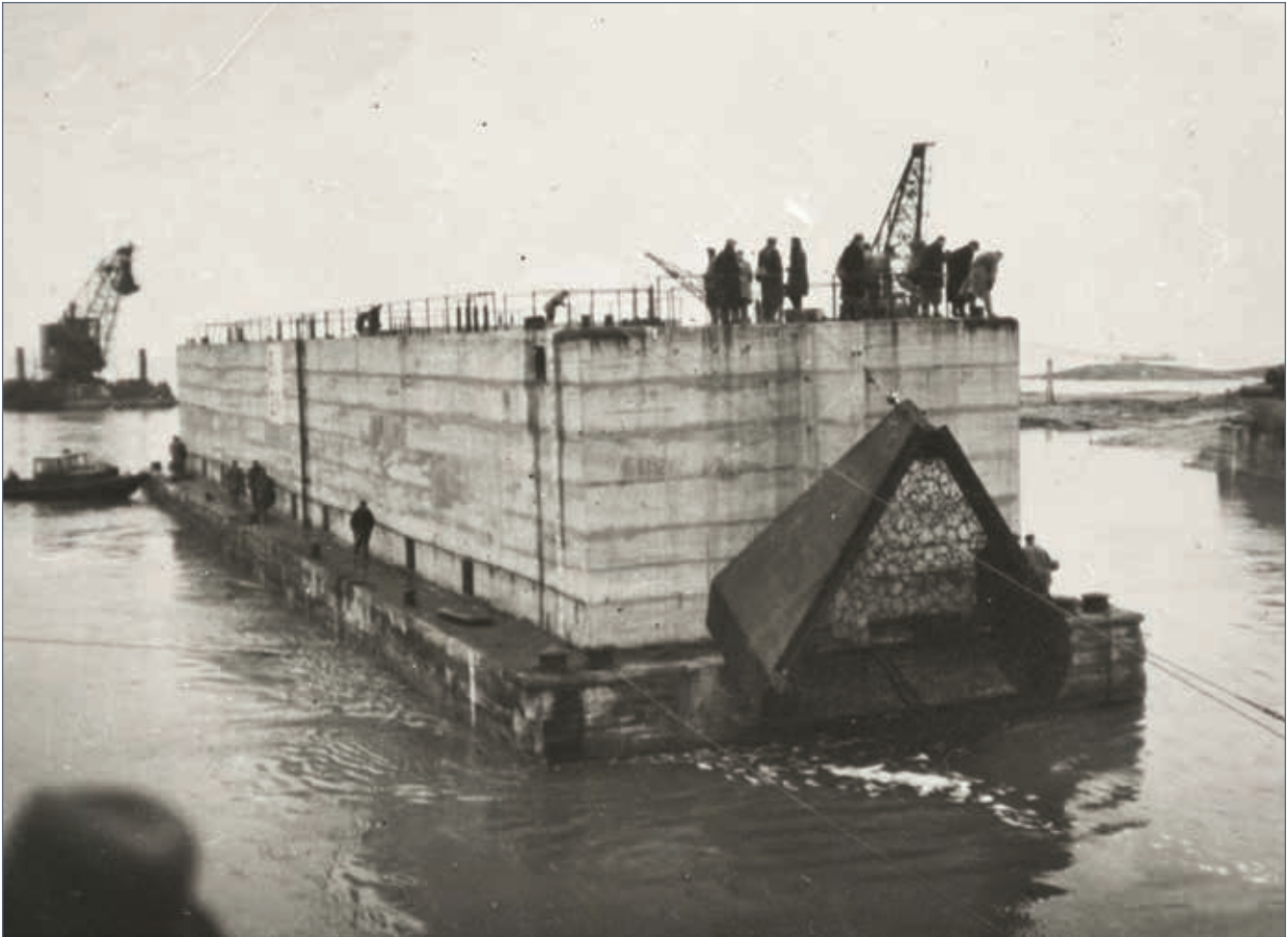
A caisson is being placed to close the last major gap on Walcheren, 1945
