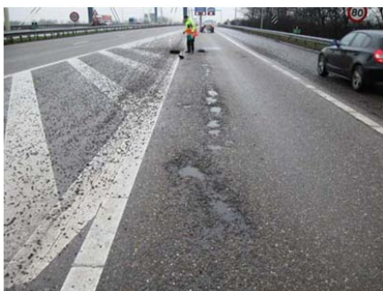
Figure 1: Frost damage on porous pavement (RWS, 2012)
