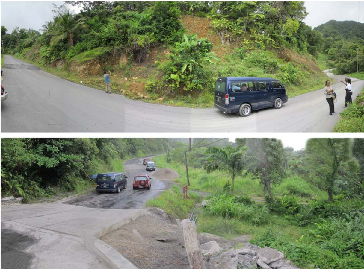
Figure 4-15: Landslide subsidence along two problem areas along the road from Canefield to Melville hall.
