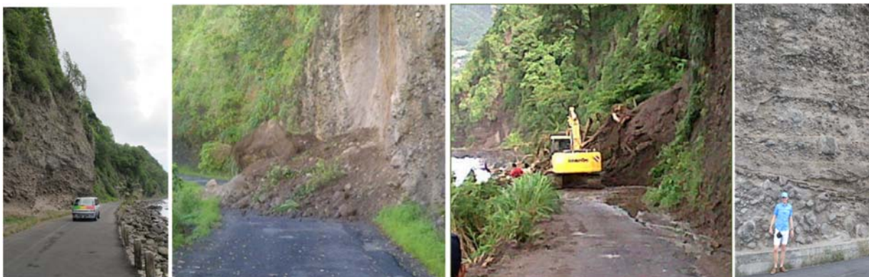
Figure 4-14: Landslide and rockfall problems in the Stowe-Dubuc area in the SE of Dominica.
