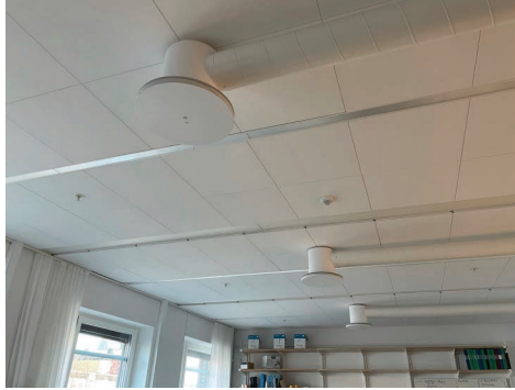
Figure 11.77 Photo of the A-building's ventilation inlet.
