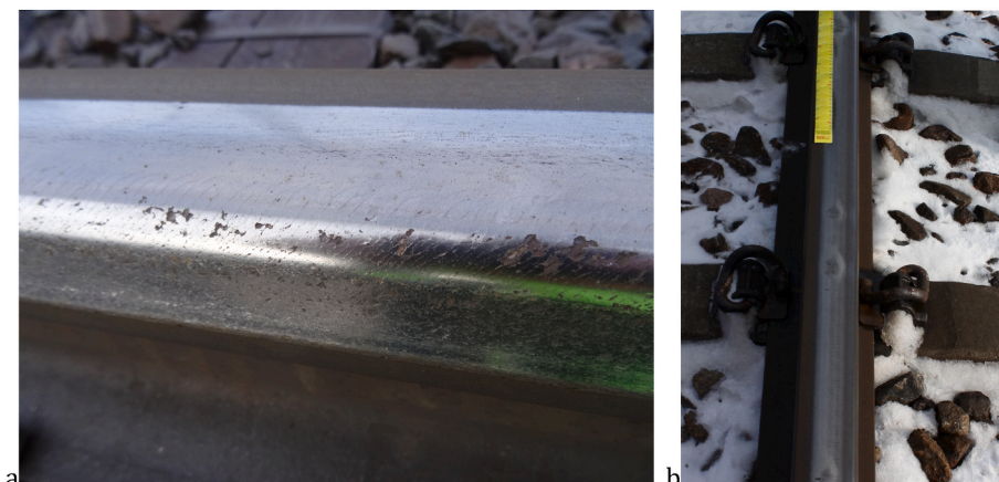
Fig. 4. a) Headchecks on the rail gauge corner. b) Squats on the railhead (right).
