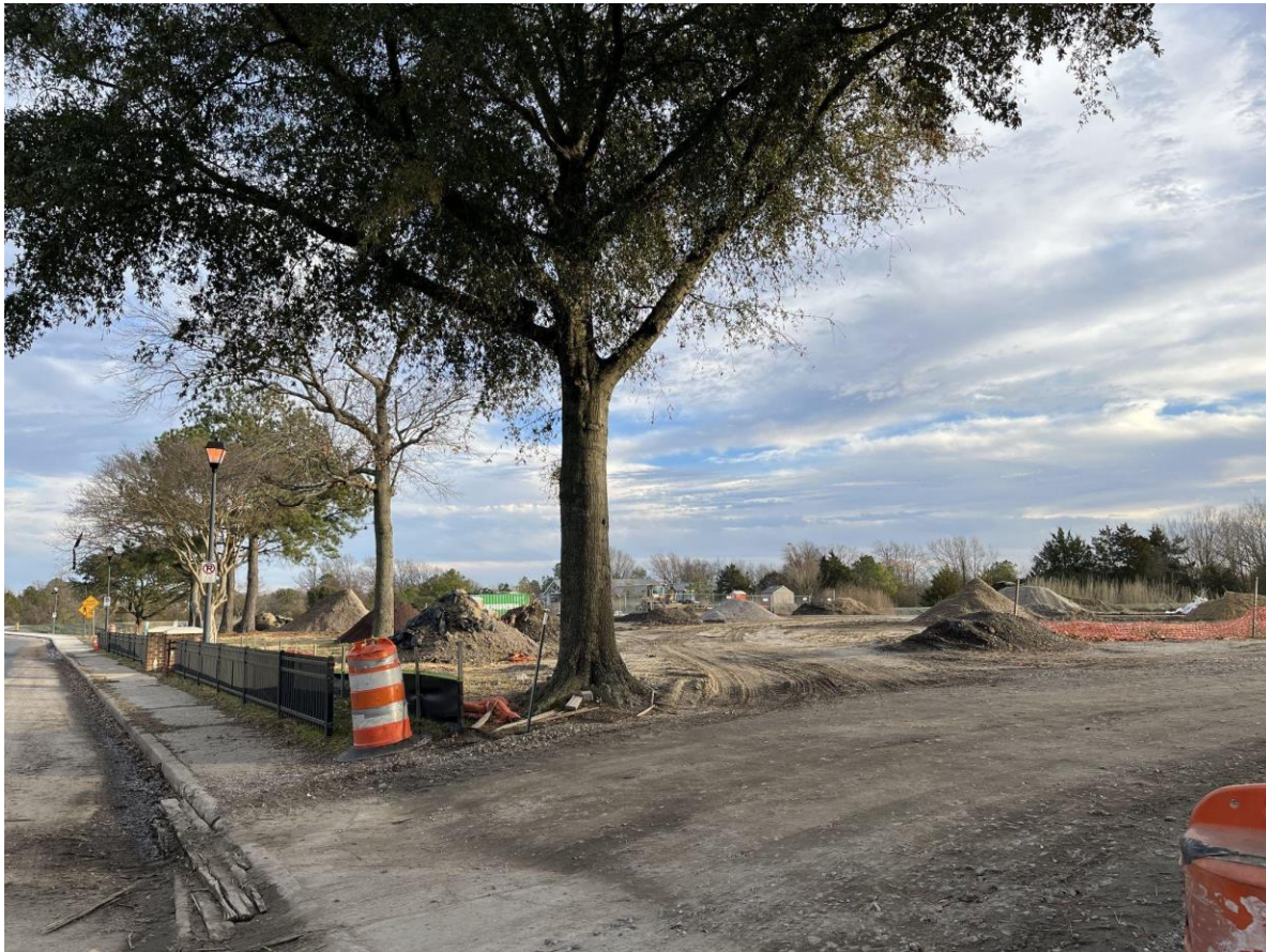
Figure 15: Construction of the Resilience Park in the Chesterfield Heights/Grandy Village neighborhoods as a part of the Ohio Creek Watershed Project. Taken by Molly Frey, January 10, 2023.
