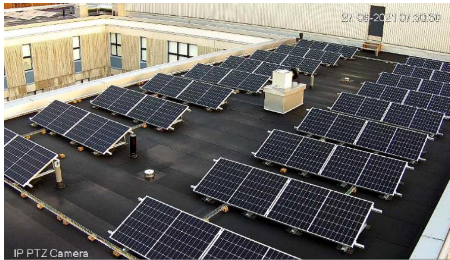
Figure 16: Roof panels with varying tilt angle setup
