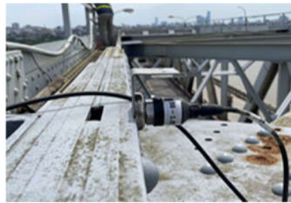
Fig. 8. One of the sensor installation position at truss node
