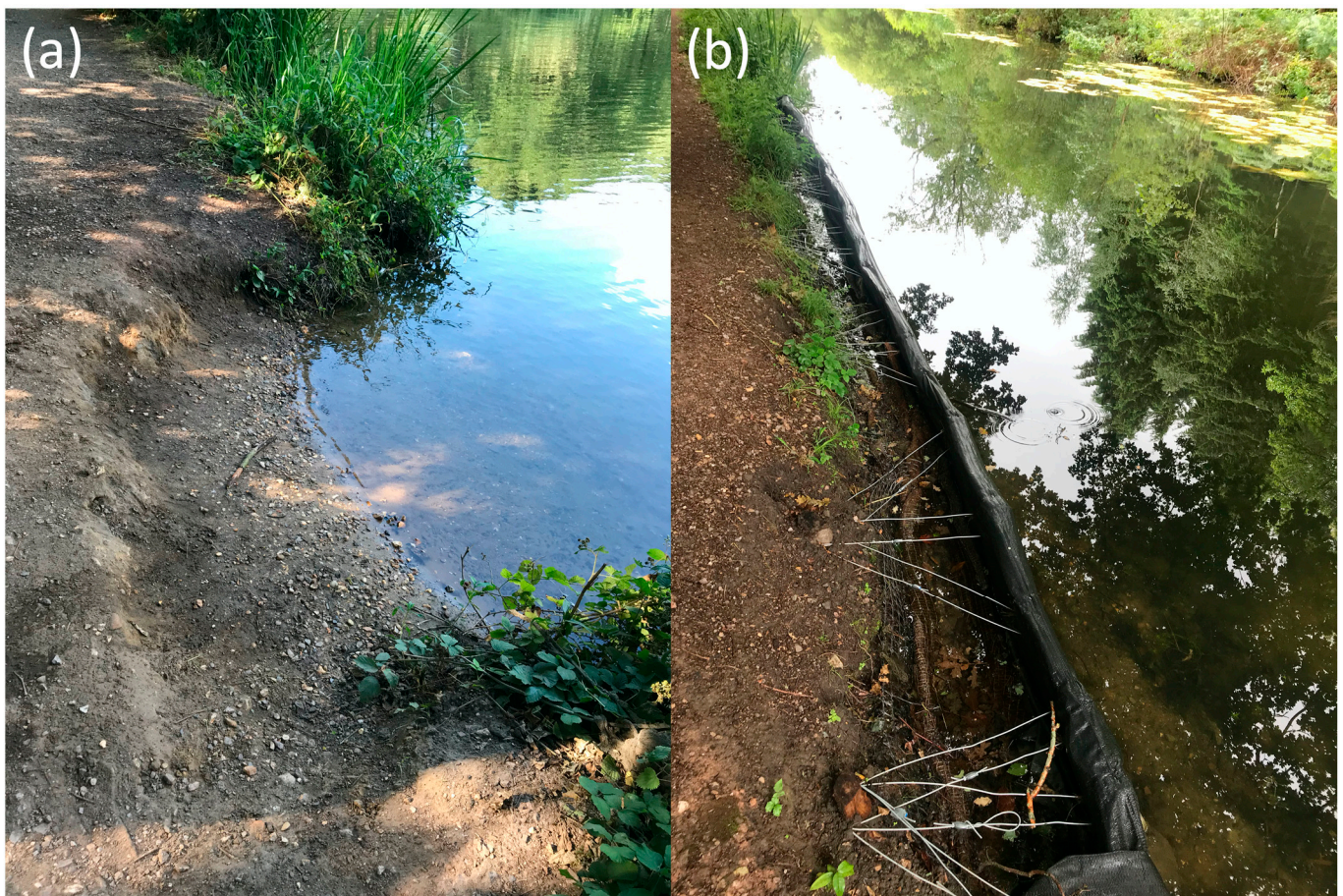
Figure 1. Illustration of engineering treatment. Photographs (a,b) were taken by Brittany Pugh. Photo (a) shows typical bank erosion, primarily caused by dogs, which is infilled using bank engineering (b). Photo (b) shows “in-progress” bank engineering. Existing above- and below-ground vegetation is removed and replaced with brush and dredged material, which is held in place by wire supports and a biodegradable mesh membrane attached to wooden posts using galvanised metal staples. Plants are then allowed to re-establish naturally. However, sometimes some vegetation remains (photo b). Note that although the soft-engineering design is standardized, the size of the area affected varies according to extent of erosion.
