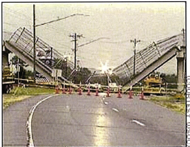
Figure 1-2: Picture of a collapsed steel-reinforced concrete pedestrian bridge in North Carolina, USA. [21]
