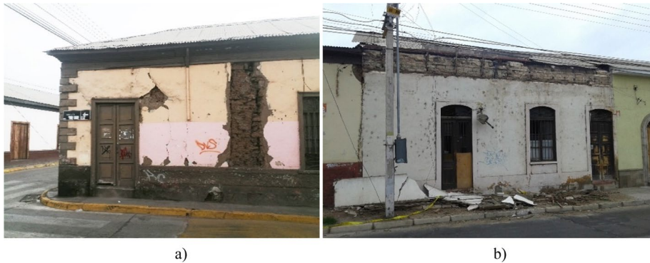
Fig. 7 a Poor interlocking connection of the adobe bricks at intersections; b impulsive nature of the roofing structure
