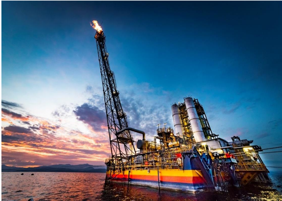
Figure 2-14: The new Kivu Watt power plant, fired by methane gas trapped deep within Lake Kivu and built by U.S. energy firm Contour Global. Werner Krug, 2015 [169].
