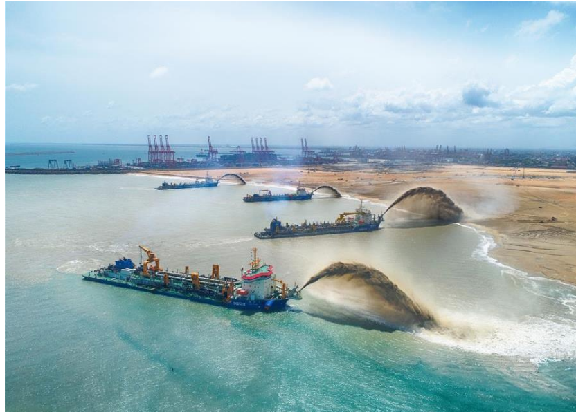
Figure 4.4 Pumping soil into reclamation area (China – Sri Lanka jointly build “Shining Pearl of Indian Ocean”, 2019)
