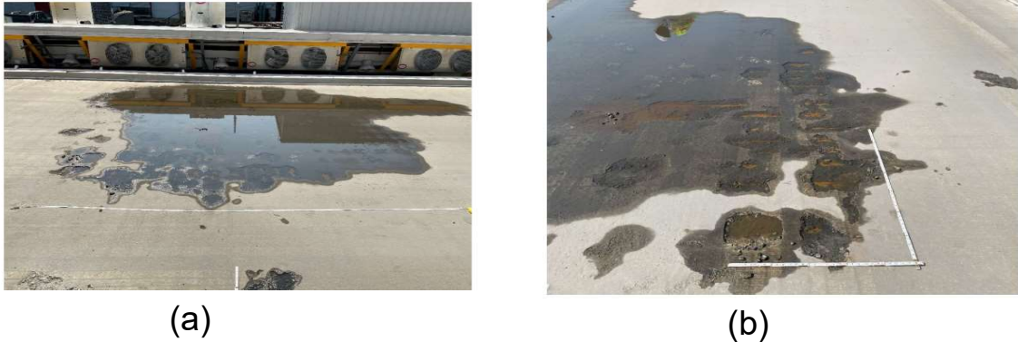
Figure 11. Images from visual inspection reports of the BEAST (a) Small to large spalls (35 SF total) looking east (b) 25 SF large spalls looking south.
