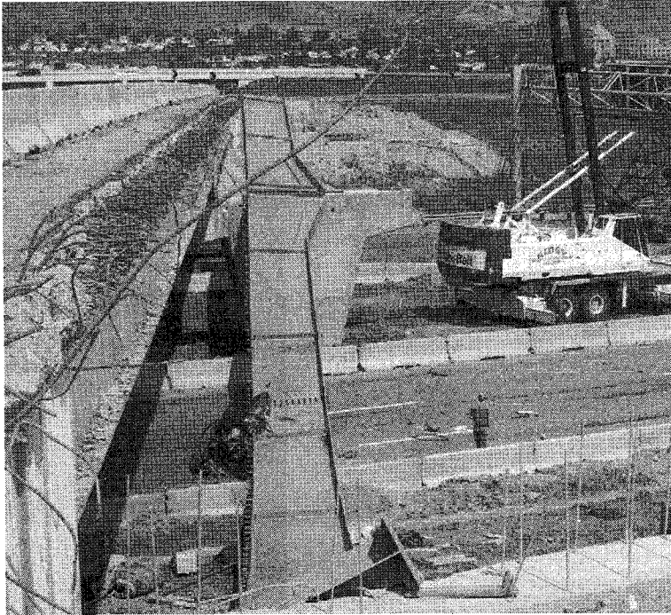
Figure 3: C-470 Bridge steel girder under construction collapsed on eastbound vehicle on I-70 near Golden, Colorado. 46
