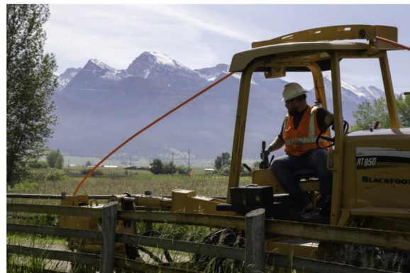
A Blackfoot Communications employee installs conduit for fiber optic cable near St. Ignace, Montana, June 2020.
