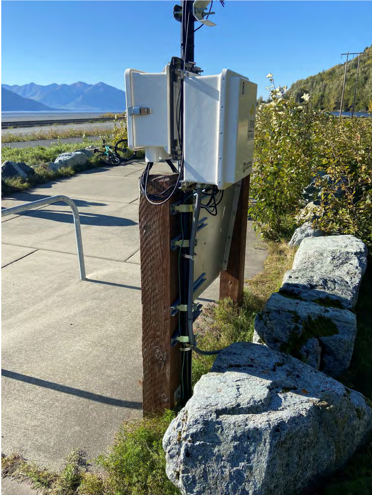
Seward Highway MP 98.5: Kalitec post mounted to informational sign along rest area of walking trail.
