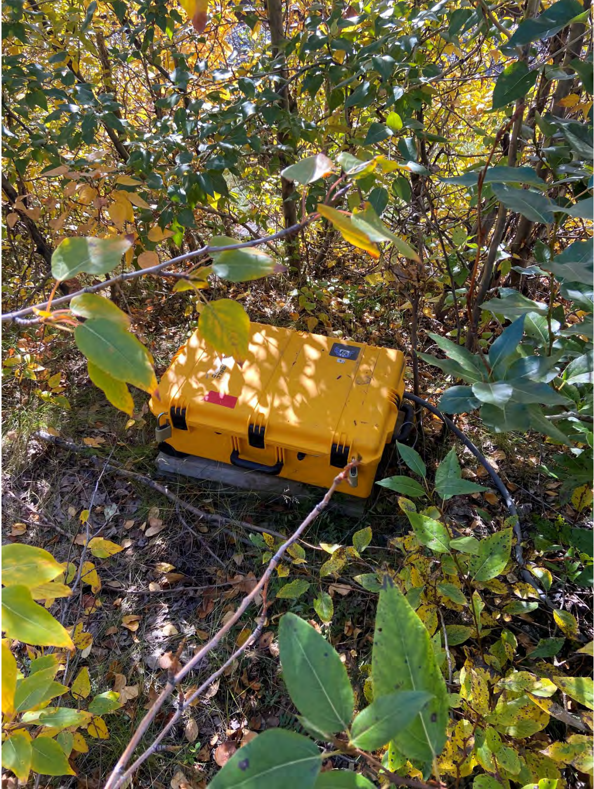
Seward Highway MP 113.5 battery box nestled snugly in wooded area.
