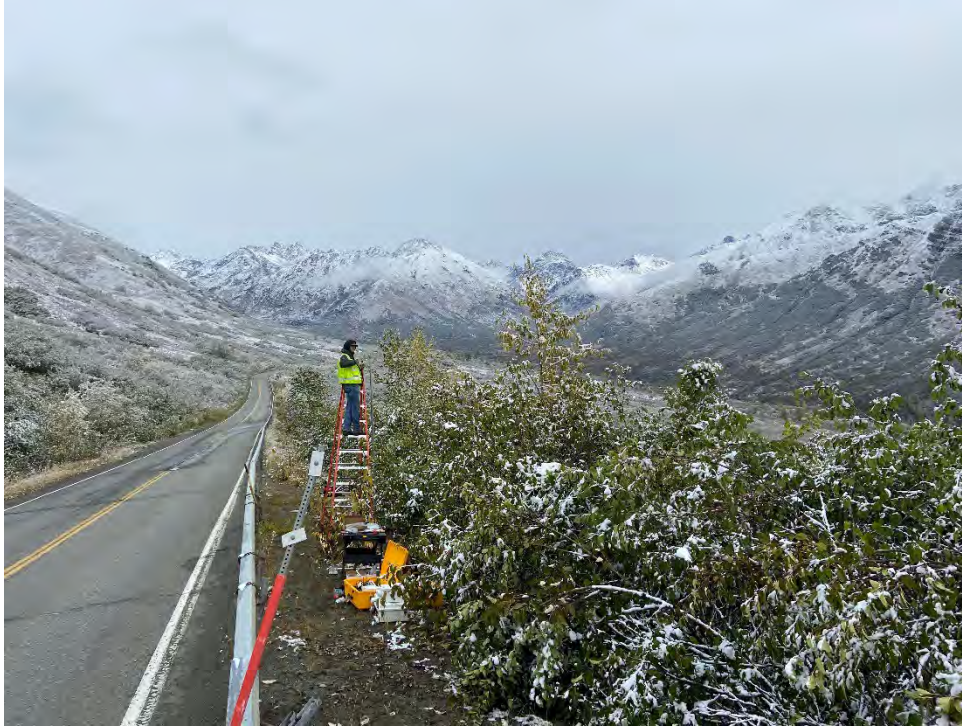
Hatcher Pass MP 15 station being installed. View looking northeast toward avalanche area.
