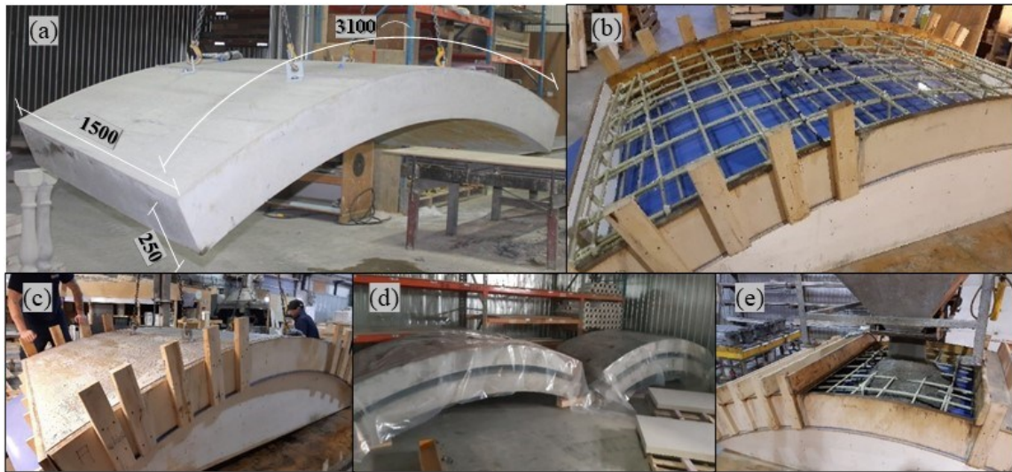
Figure 6.1 (a) Geometry of tunnel segment specimens (dimensions in mm); (b) fabricated cage inside formwork (7G#5F); (c) casting of the specimens; (d) demolding; and (e) curing.
