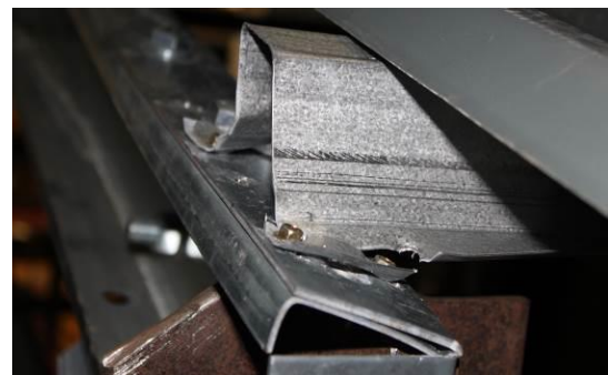
d) Failure of purlin connection and deformation of the gable-frame rafter
