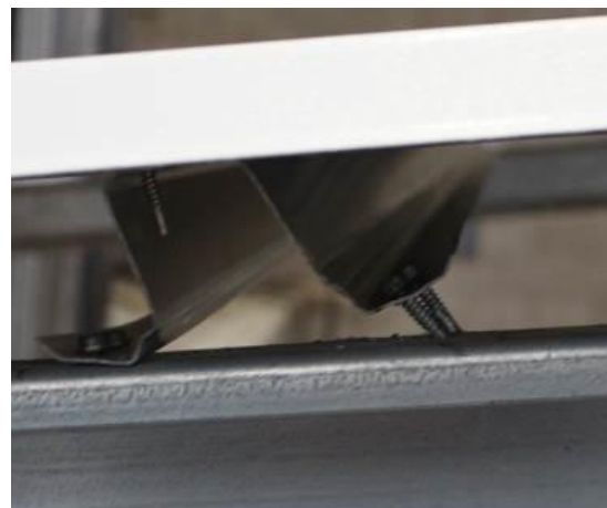
b) Failure of purlin-to- end-rafter connection
