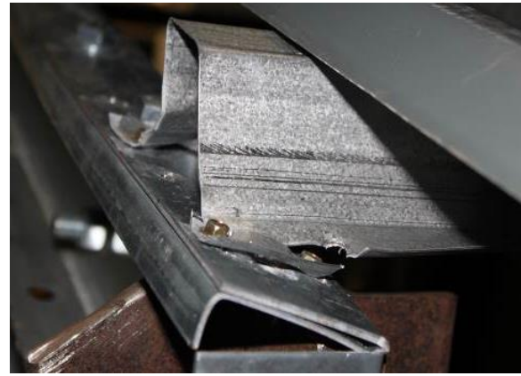
b) Failure of purlin connection and deformation of the gable-frame rafter
