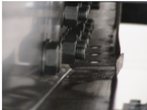
a) local buckling of the bottom flange and lip close to outer line of bolts
