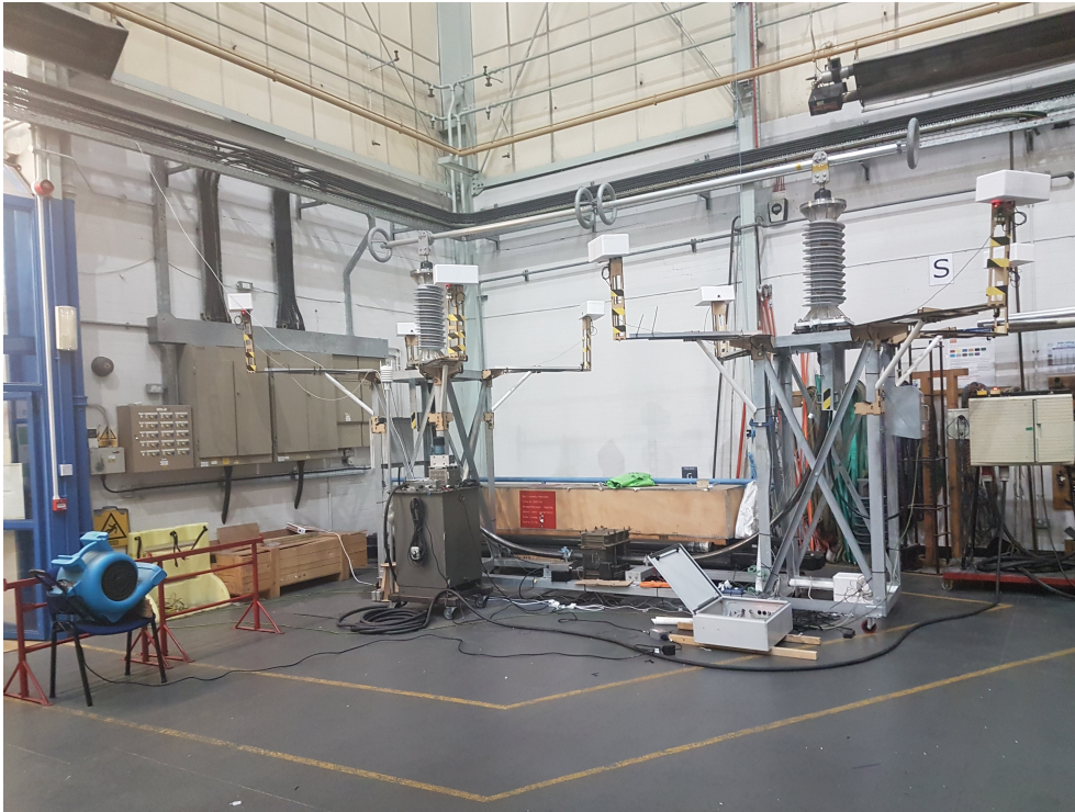
Figure 4.5: The full cable sealing end experimental rig
