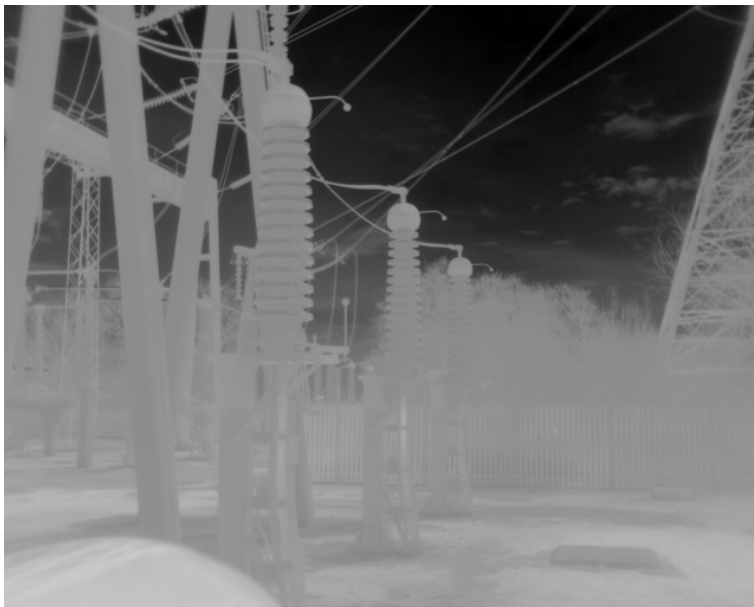
Figure 1.3: A set of three cable terminations, as observed by a thermal camera, in a National Grid Substation
