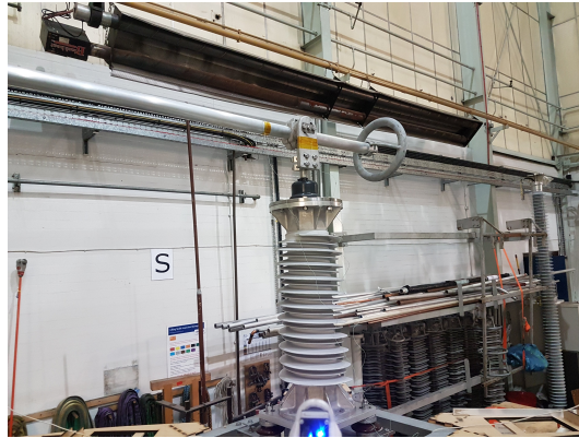
Figure 4.2: A cable-sealing end in the B23 high-voltage laboratory, as seen from the approximate perspective of camera 8.
