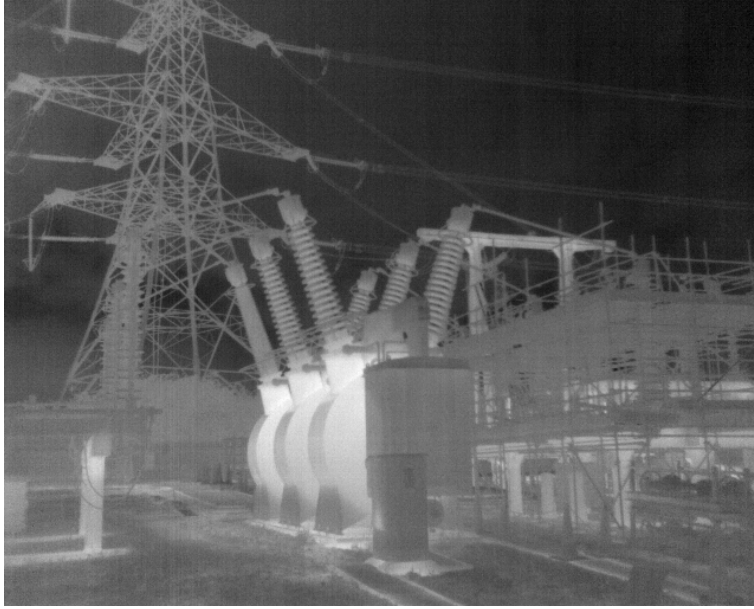
Figure 1.2: A circuit-breaker, as observed by a thermal camera, in a National Grid Substation
