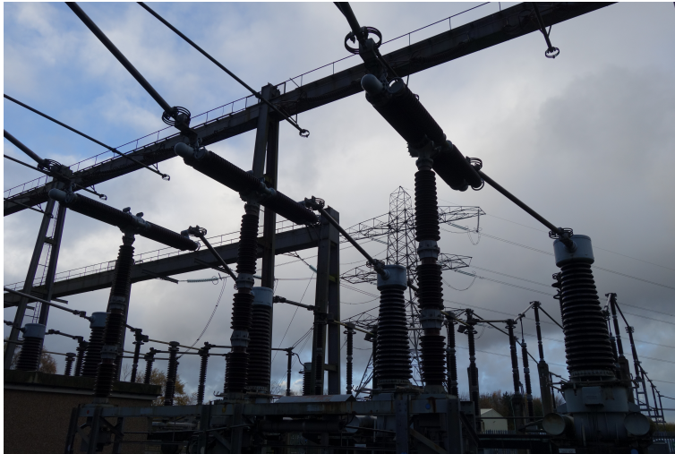
Figure 1.1: A National Grid Substation in North-West England
