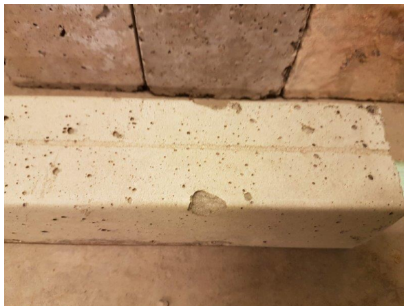
Figure 4.10: Bubbles observed in grout finish
