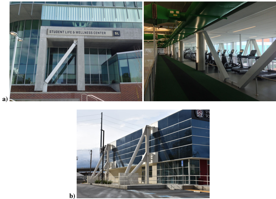
Figure 1.2: a)UVU Student Life Centre, steel frame built retrofitted with 132 BRBs, some in chevron arrangement.b)Stratford School, external braces connected to the same plate Image from: CoreBrace (2021)
