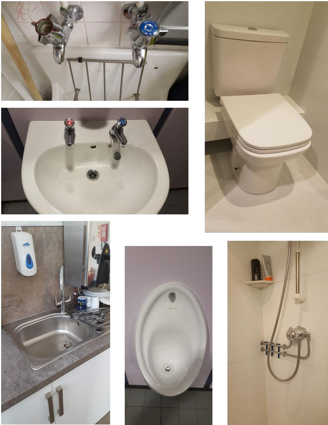
Figure 5-3 Examples of sanitary appliances in the case study buildings
