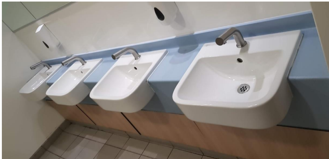
Figure 5-29 Sensor water taps in Hugh Nisbet Building
