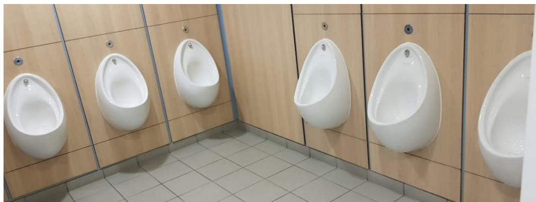
Figure 5-30 Sensor urinals in Hugh Nisbet Building
