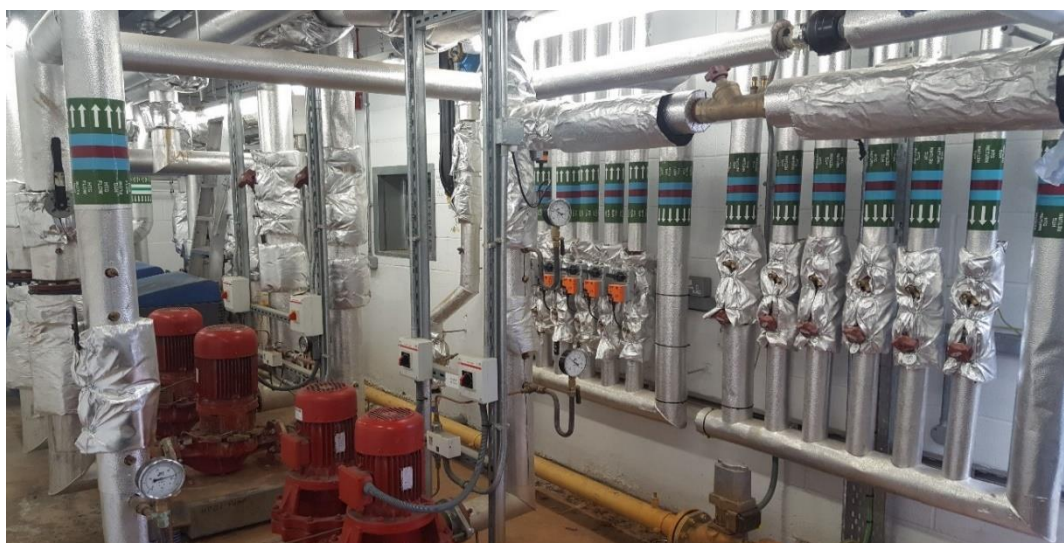
Figure 5-24 The plant room in the Postgraduate Centre
