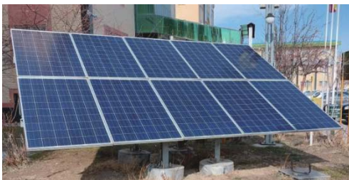
Fig. 25. BP SX3190 solar panels which used in the experiment.
