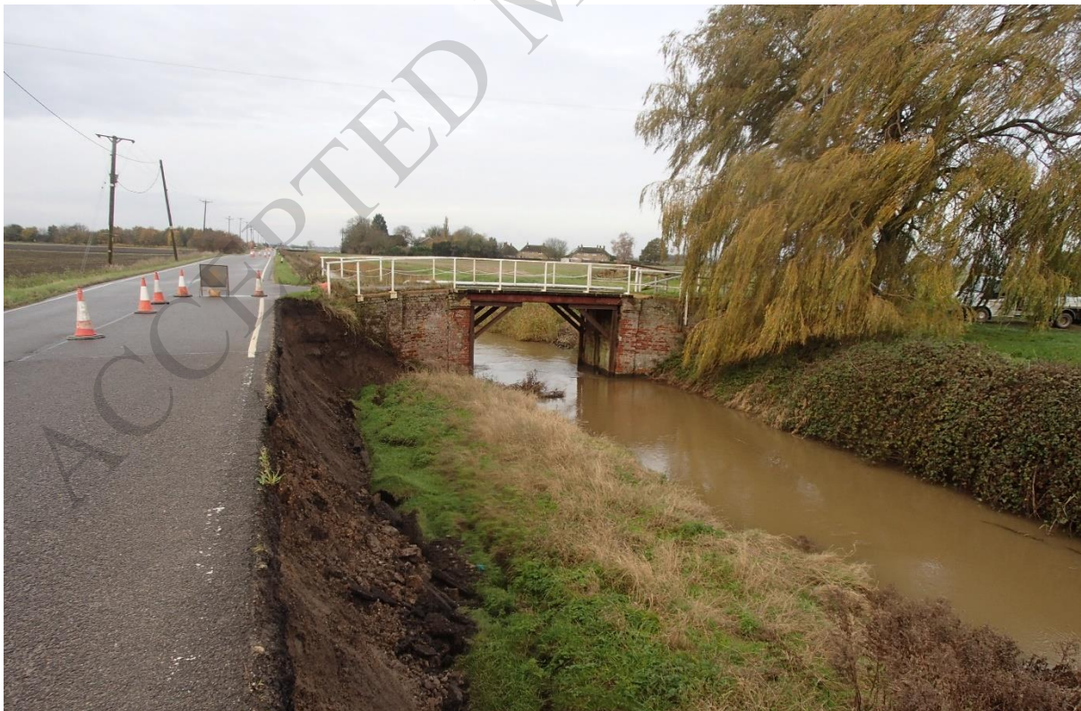
Figure 5 Landslide in large ditch adjacent to road, causing road subsidence and closure for repairs in Autumn 2019. Fodderdyke bank, Midville © Mark Heaton LCC
