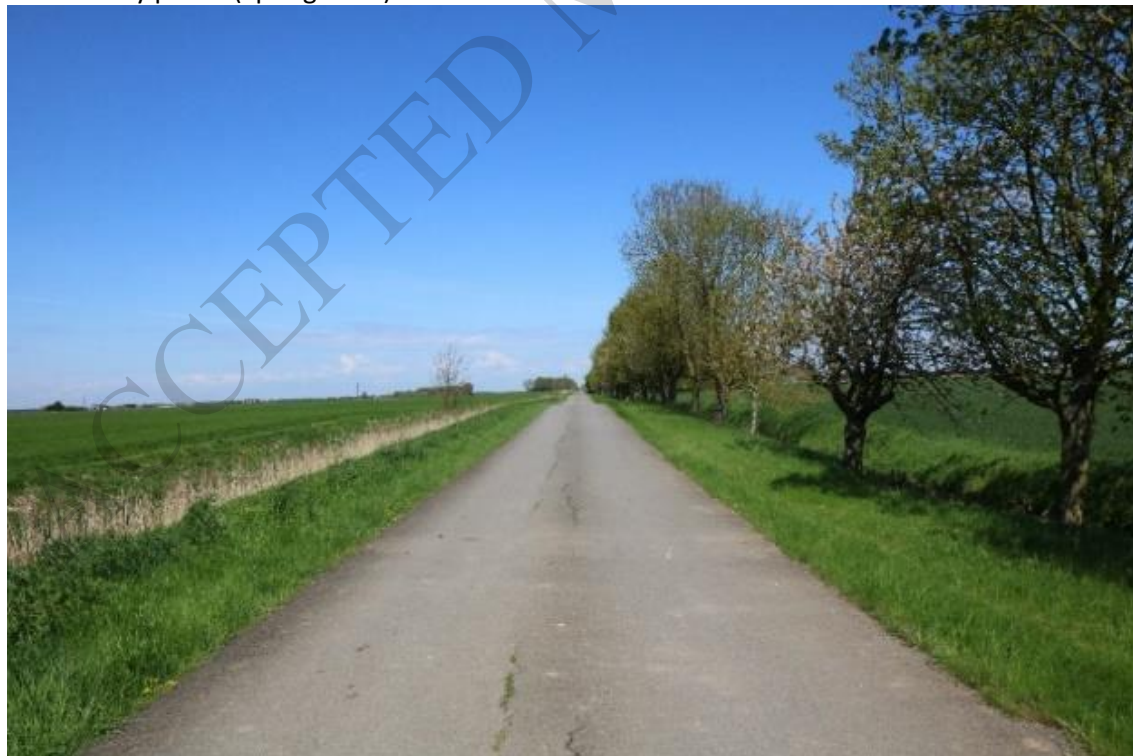
Figure 14 Amber Hill. Top: Geological map. Bottom: Photo taken May 2018 showing longitudinal cracking along the centre of the road. BGS © UKRI 2018
