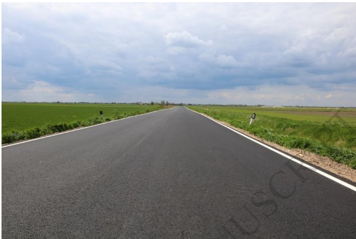
Figure 23 Fodderdyke (eastern end of Fodderdyke) following resurfacing using the new recycling method (May, 2018) BGS © UKRI 2018
