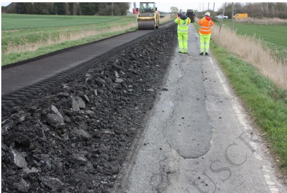
Figure 21 Shaping and compaction of the pulverised existing road surface at Fodderdyke Bank (March, 2018). © Mark Heaton LCC
