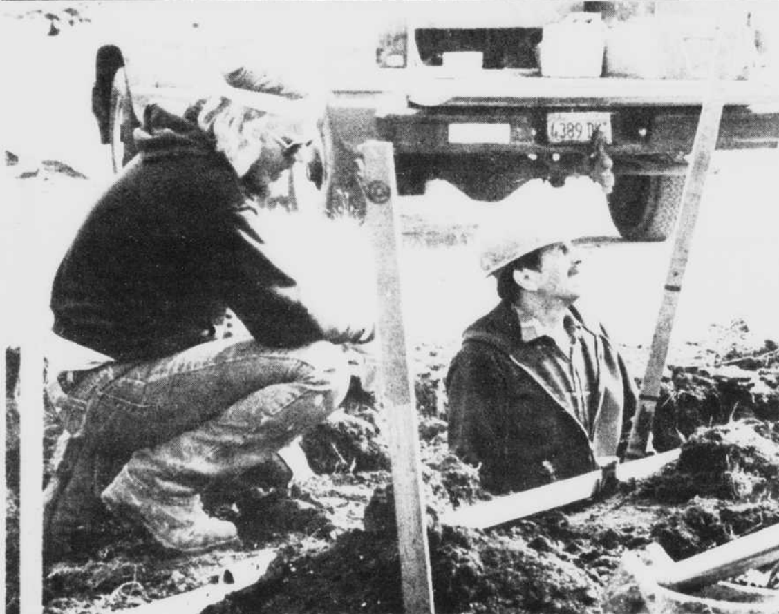
Busy at work installing a storm sewer are Bill Archer (right) and Ron Felty. Their work is a part of construction that is going on to move Anthony Drive north. This particular site was manned by Cross Construction Company.
