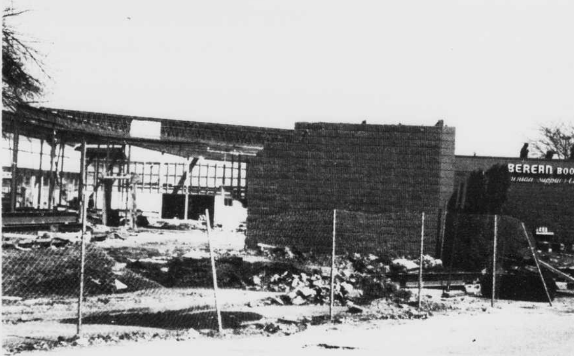
Work is progressing on many construction projects in west Champaign this month, with the weather cooperating to the utmost. This picture was taken at Country Fair Shopping Center, which is undergoing a complete redesign.
