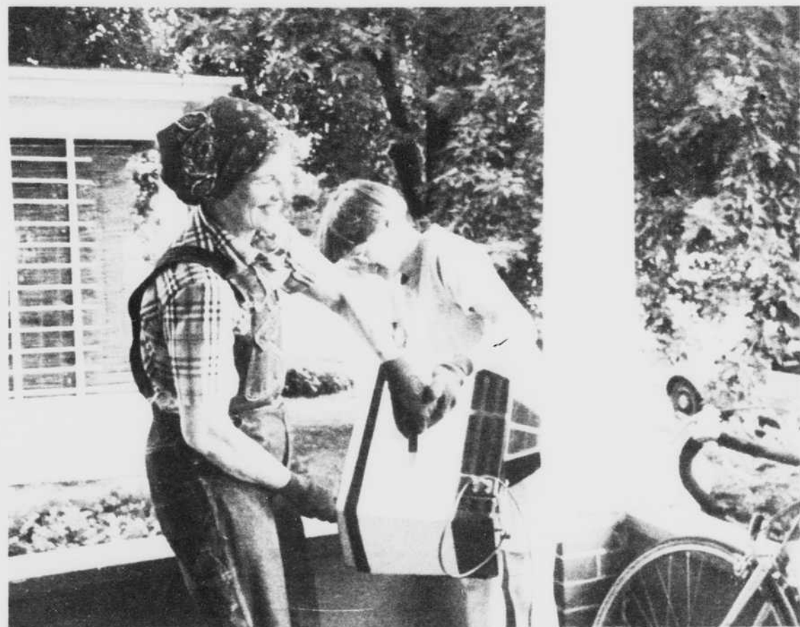
Hey, this is heavy! Ellen McDowell and Frances Drone-Silvers lift a TV set on the porch of the Catholic Worker House at 317 S. Randolph, which volunteers are remodeling. They hope to have the work done before cold weather comes this fall. Photo by Joan Doaks
