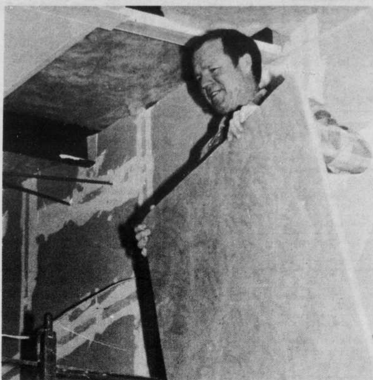
Ron Wilson installs insulating panels to ensure students and faculty a warm winter in the Annex. Work on the Annex is still underway and Business Manager Don Moran announced this past weekend that classes would not meet there today, as previously anticipated. Moran cited weather and delivery of building materials for the delay. Although the date has not yet been firmly set, January 31 should see classes meeting in the new building.
