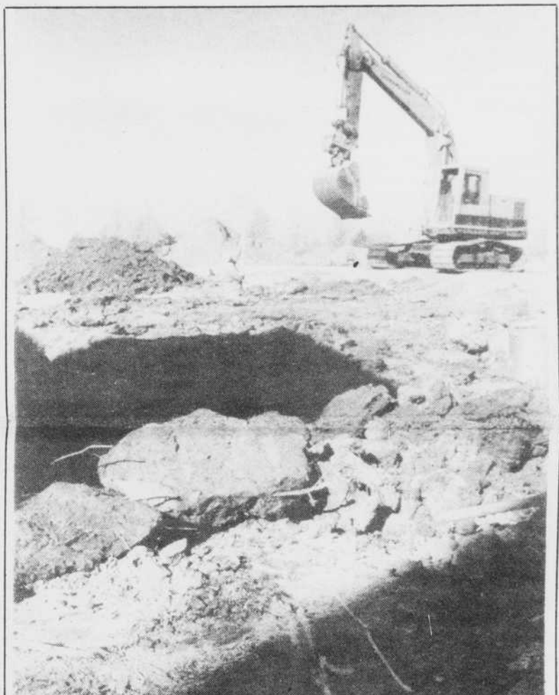
Construction continues on Parkland's Planetarium and Performing Arts Center. The construction, which began last fall, is scheduled to be completed in 1987.
