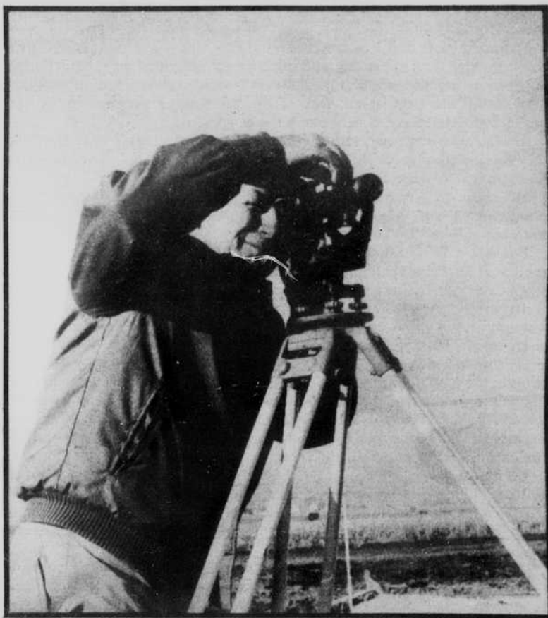
Photo by Jon Sivier A worker for the C. A. Petry Company surveys the site where Parkland's new maintenance building will be built. The building will be located on the west part of the campus.
