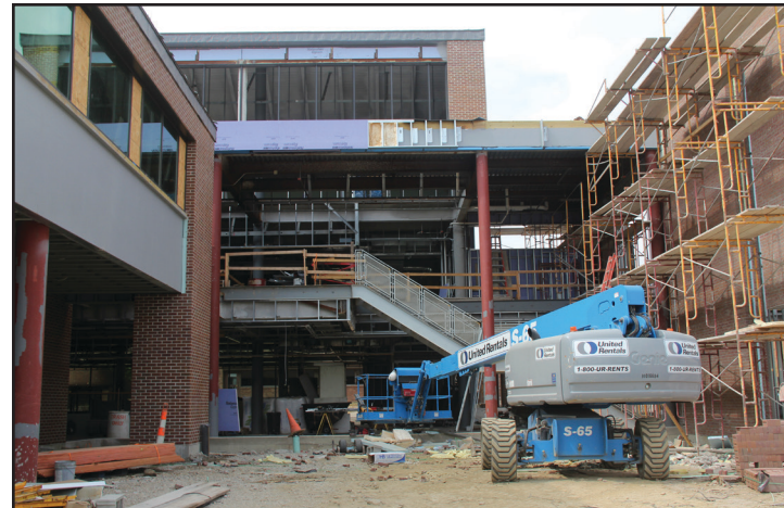
A view of the new Student Services Center, to be completed in the spring of 2014.
